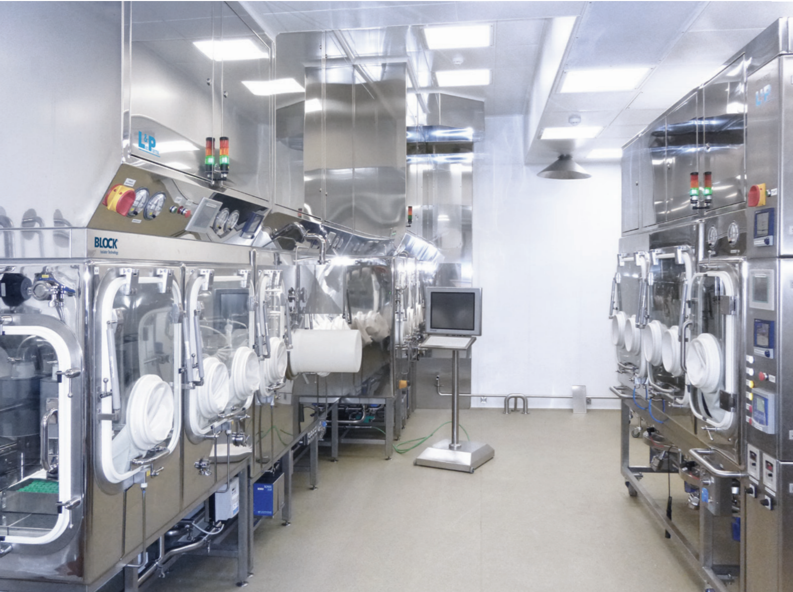
Isolator for filling of cytotostatics into bottles, inserting and unloading bottles into / from the lyophilization device and closing the bottles, RUE "BELMEDPREPARATY", Belarus
