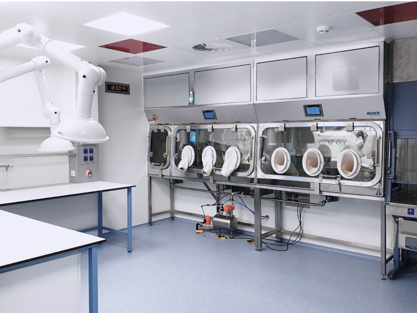
Negative pressure isolator for protect of the personal, processed material API, light sensitive, humidity sensitive, Synthon, s.r.o., Czechia
