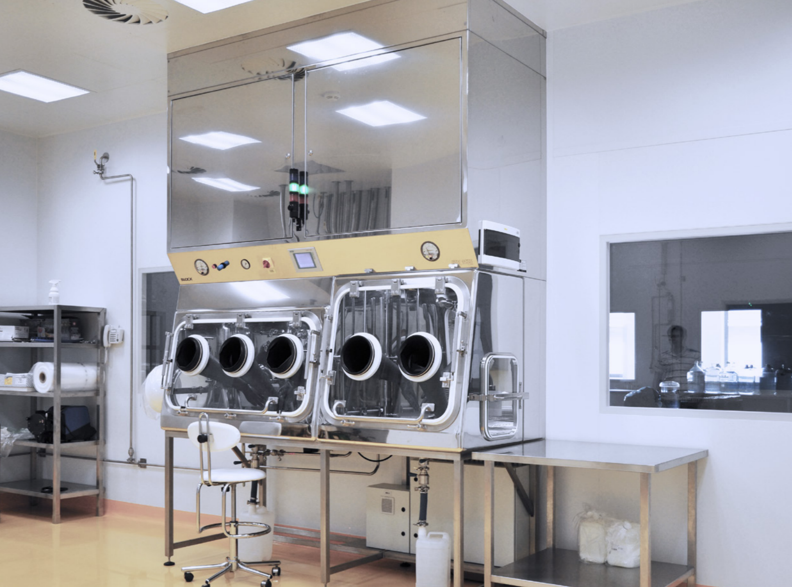
Isolator for the handling with vaccines and transfer to formulation boilers, Biotechnological Hall (Bioveta Tech Hall), Bioveta, a.s., Czechia
