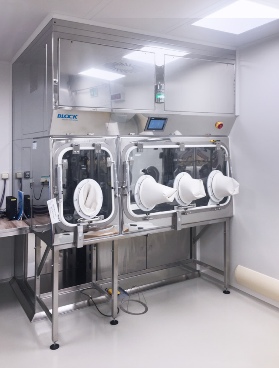
Negative pressure isolator for handling with infectious material, Praha Vaccines a.s. / NOVAVAX CZ a.s., Czechia
