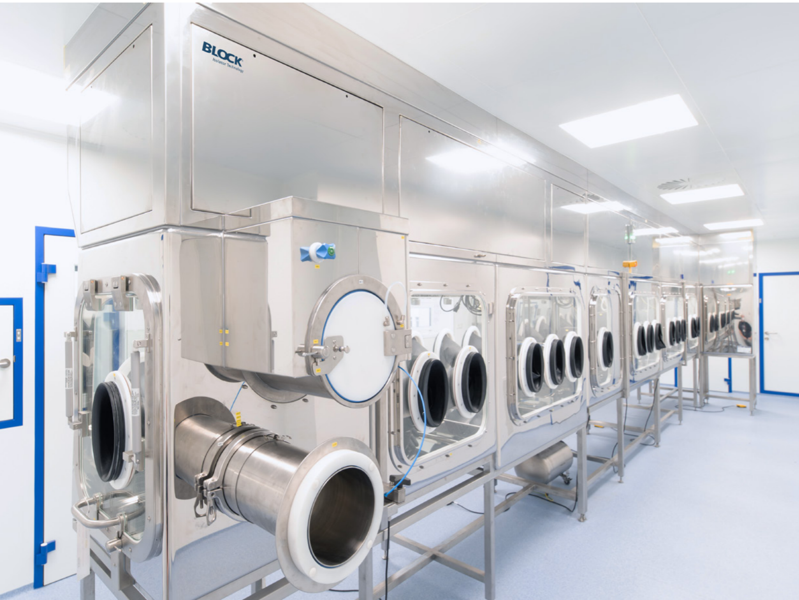
Manufacturing isolator with turbulent flow, Cayman Pharma s.r.o., Czechia
