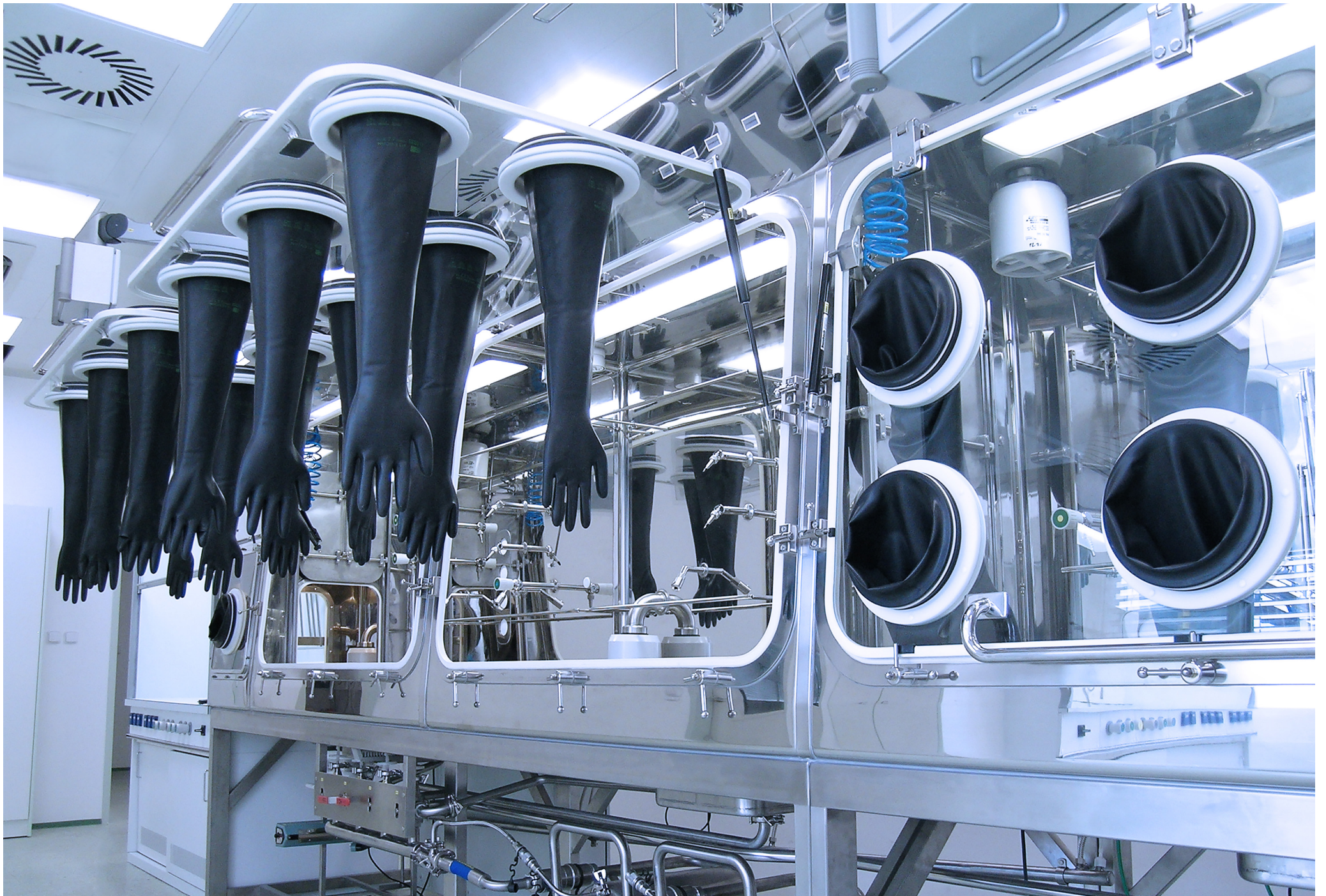
Isolator for working with hazardous materials | Zentiva Group a.s. | Prague, Czech Republic
